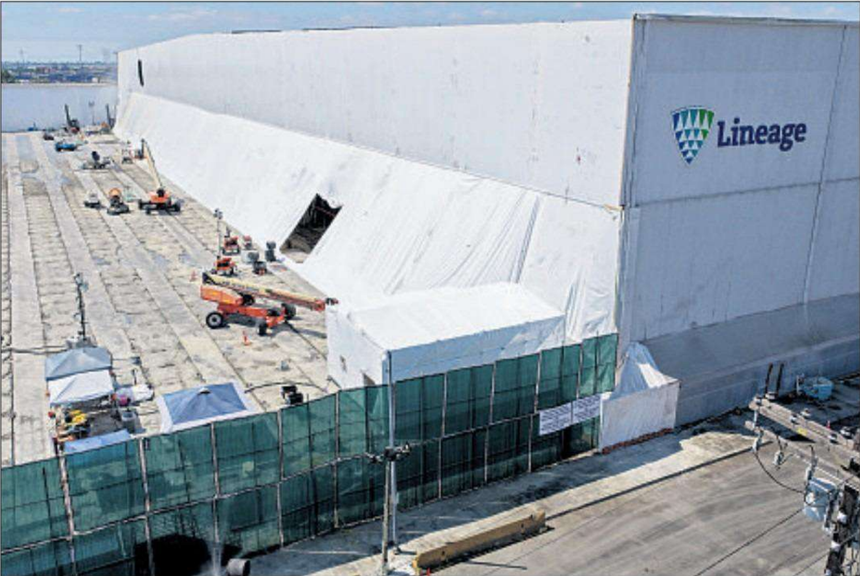
IN BOYLE HEIGHTS, crews continue cleanup efforts after a June blaze engulfed a cold storage warehouse.
